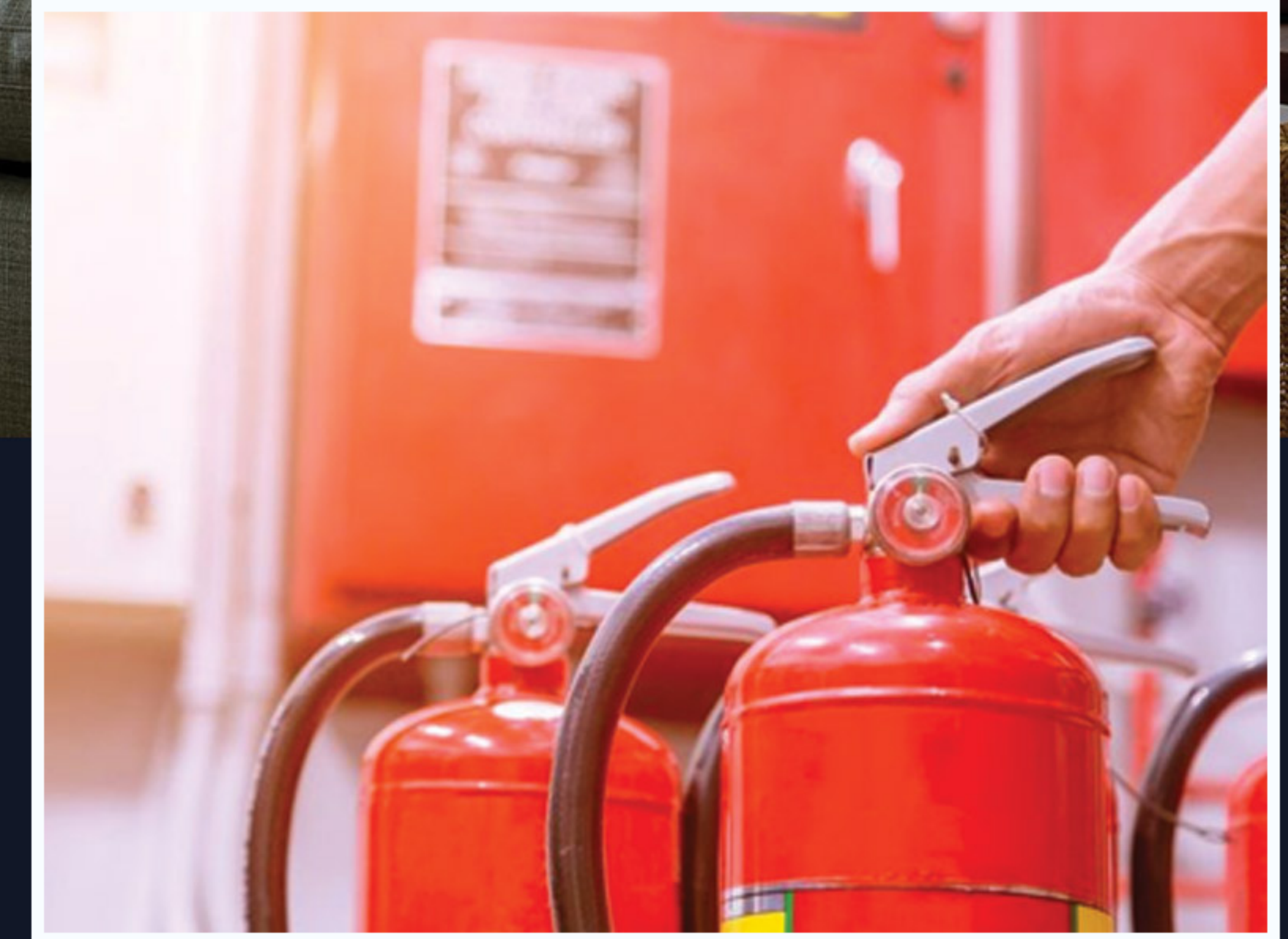
FIRE FIGHTING SYSTEM
